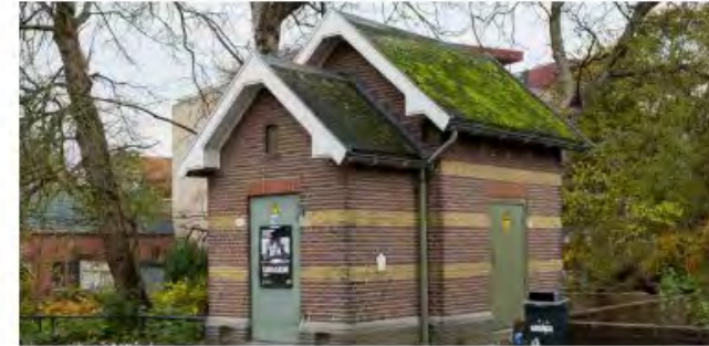
MS-MS station (3-23kV)
